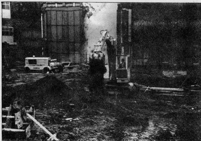
The foundations of what will become IC's sports centre— completion is expected by June 1968. Photograph by D. Ormiston
