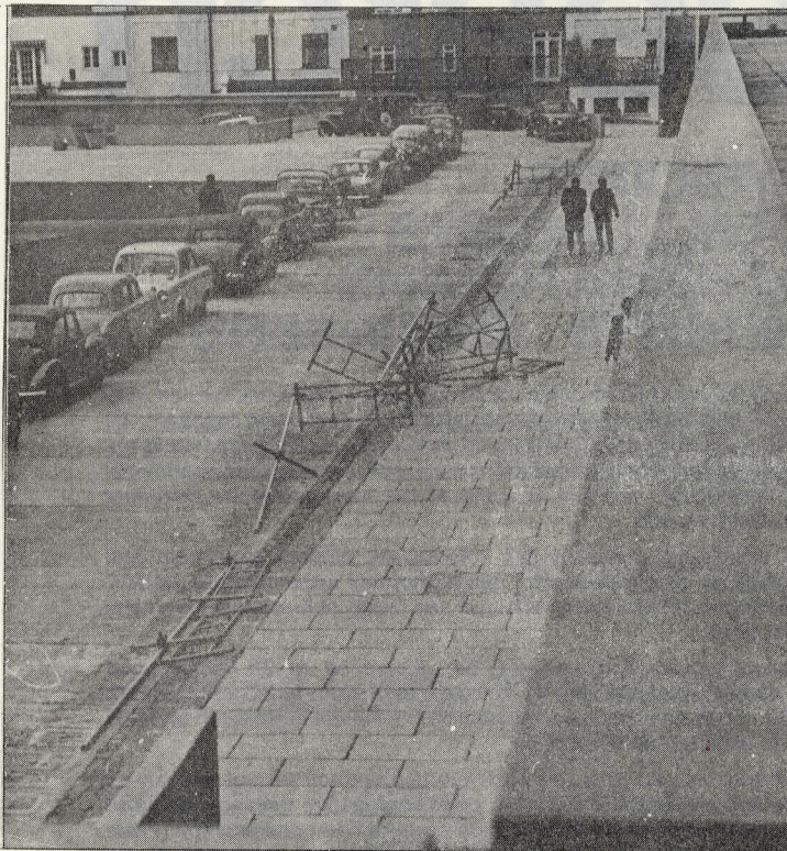
A divergence of opinion over the advisability of scaffolding in front of Southside led to this pile-up early Friday morning.
