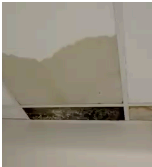
A leaky roof in 15B Princes Gardens. Idrees Mahmood
