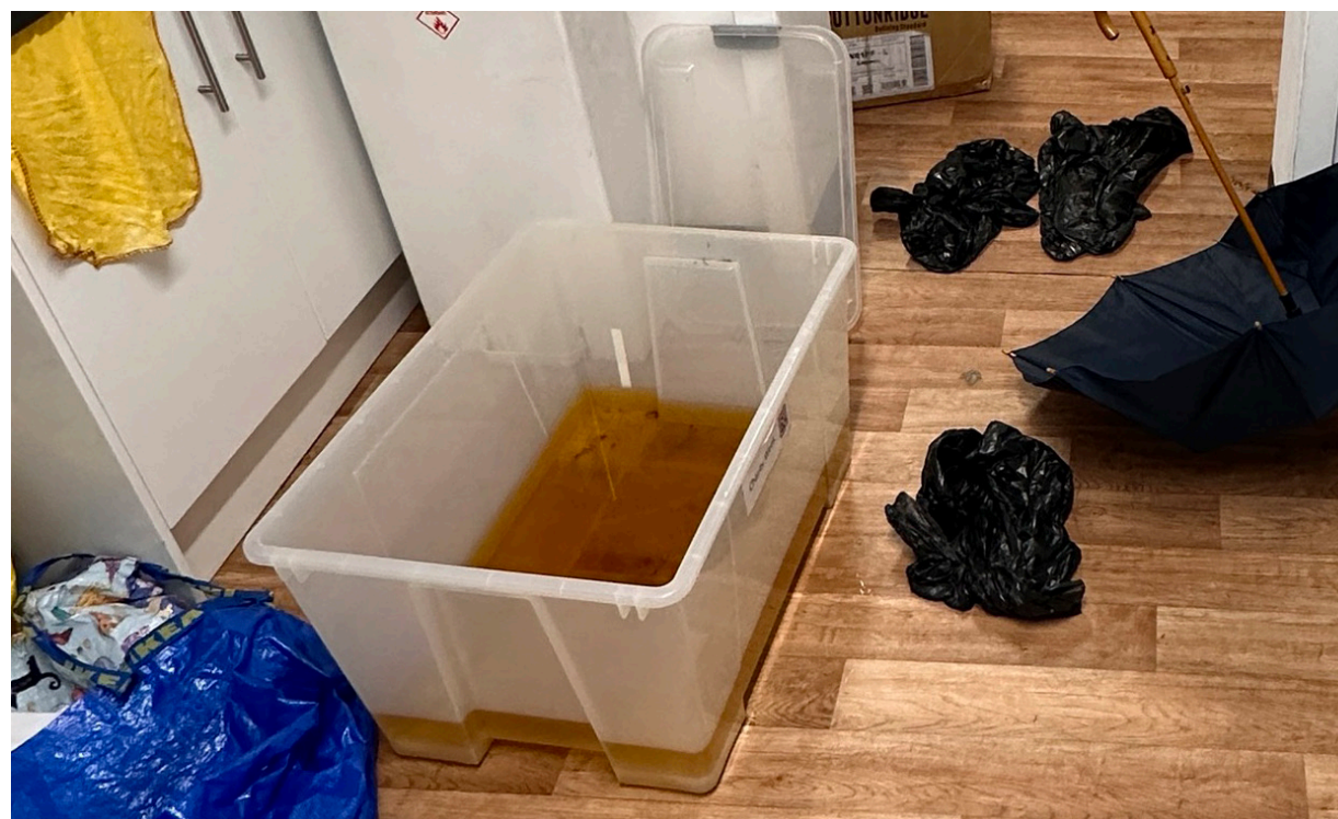
This suspicious liquid isn't urine, but instead the water collected from a leak in 14B Princes Gardens. Idrees Mahmood
