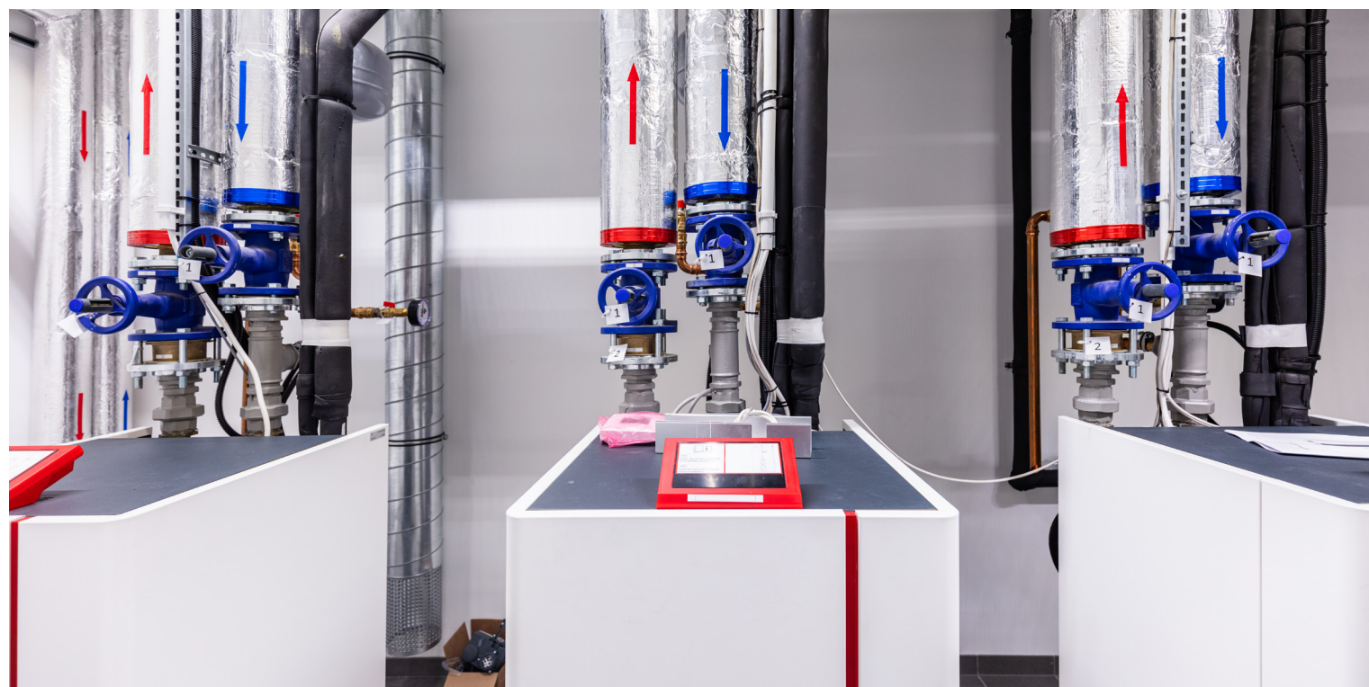
Heat pump room
