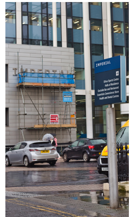
Construction workers were on campus this week to update College branding. Walt Gao for Felix
