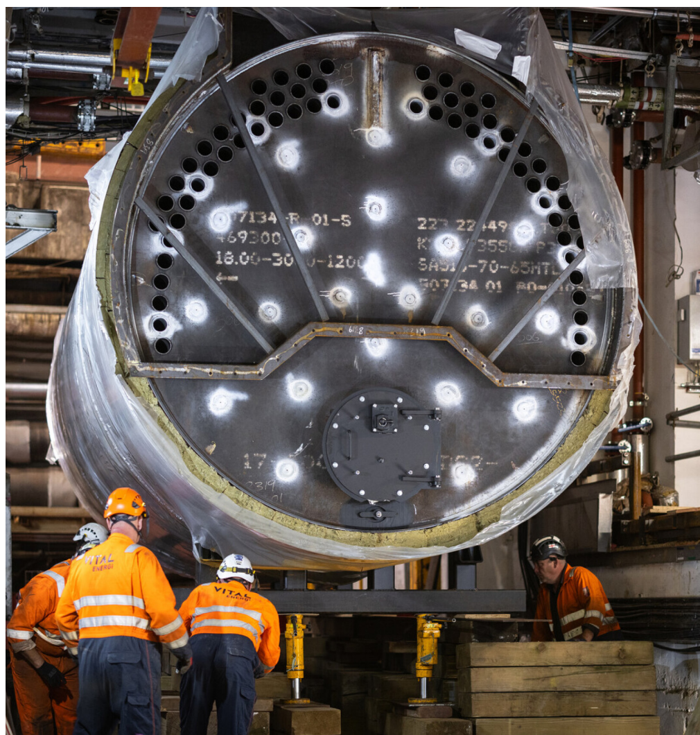
One of three new boilers Imperial is installing as part of its effort to reach net zero by 2040. Imperial College London
