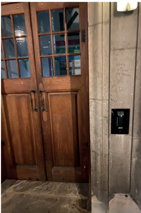
The West Basement entrance, unlocked at 10.24pm, three days after the break-in
