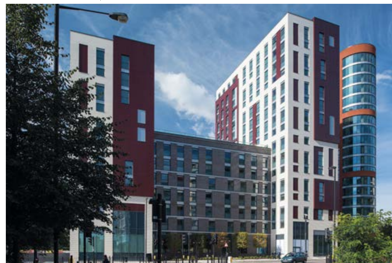
Woodward Buildings continues to have cladding that has failed fire safety tests // Imperial
