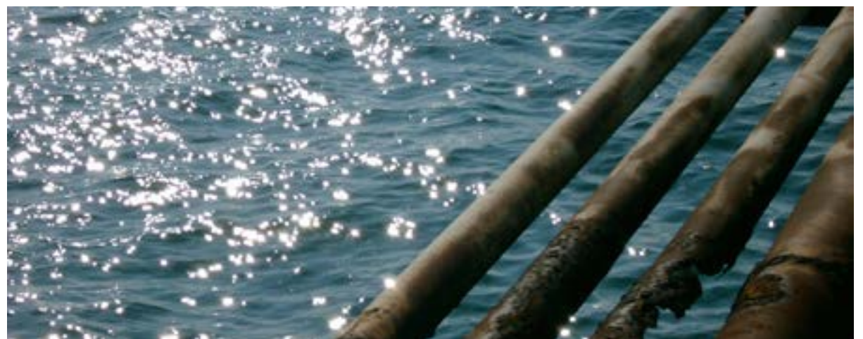
Corrosion of pipelines has been a technical challenge for Qatari industries. Photo: knovel.com
