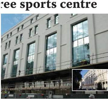
The new sports centre as it stands and (insert) an artists impression of the finished centre
