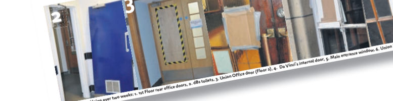
Damage to the Union over two weeks: 1. 1st Floor rear office doors, 2. dBs toilets, 3. Union Office door (Floor 3), 4. Da Vinci's internal door, 5. Main entrance window, 6. Union Bar door
