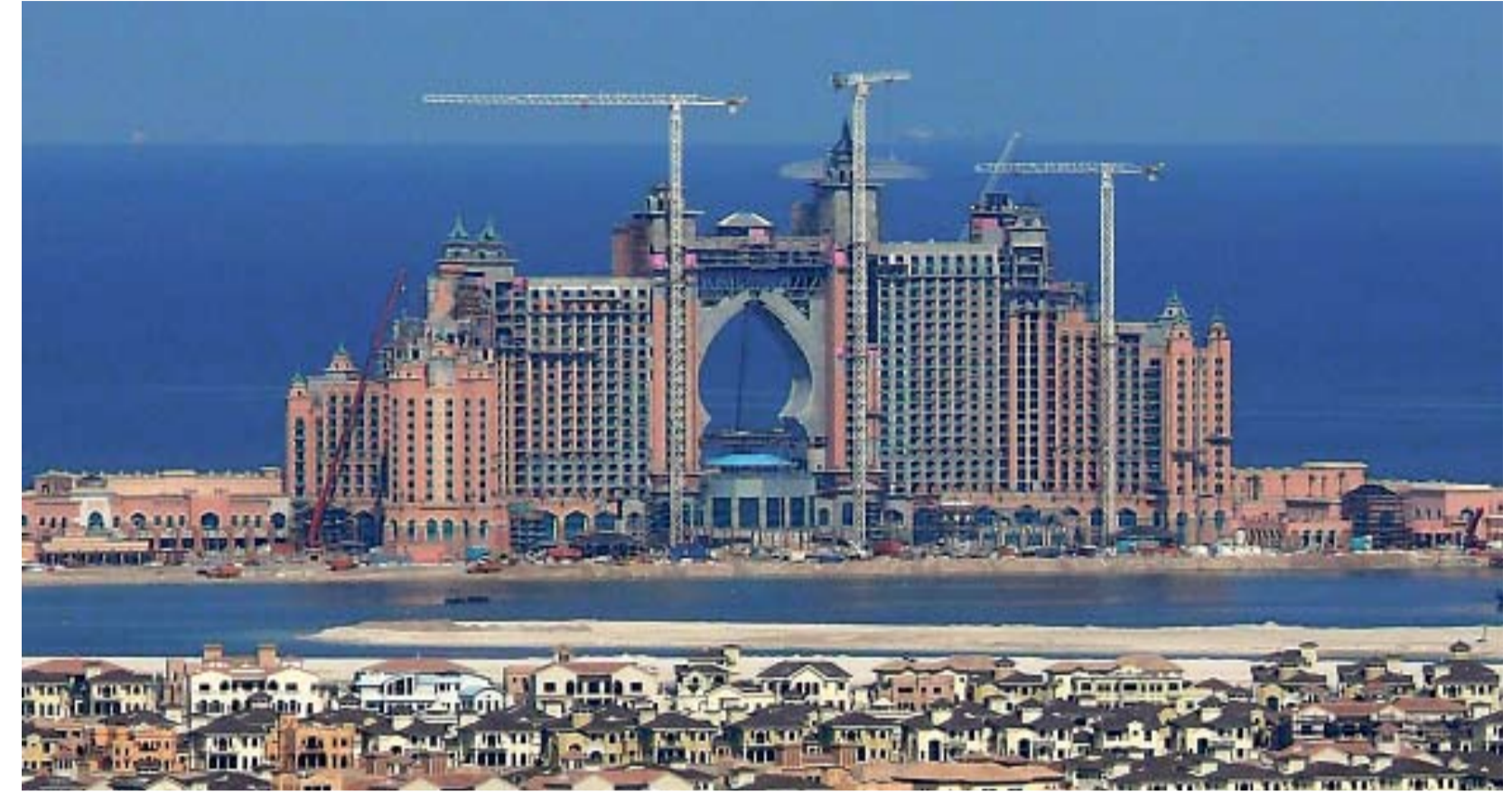
Dubai has received criticism from its people and from international organisations for the Atlantis hotel, the latest in a string of lavish projects
