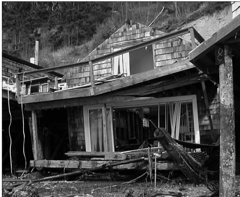
A defective house. Or should that be Defected?
