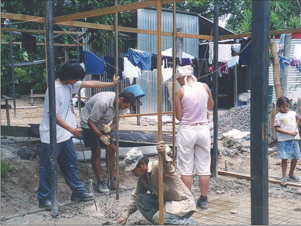
7. Lay the slab, 'tamping' as you go to remove any air voids
