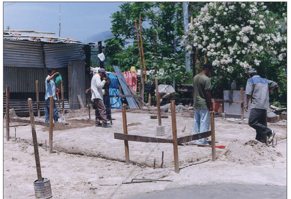
4. Recompact (by hand) the soil that you have excavated. Nurse your blistered, minging hands. Set out the site and begin to dig trenches
