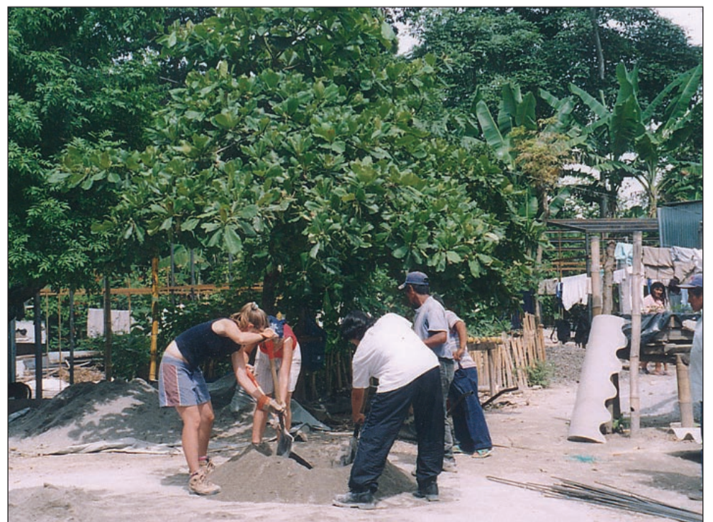
6. Mix concrete for the floor slab (if you have enough water from the previous night's rain)
