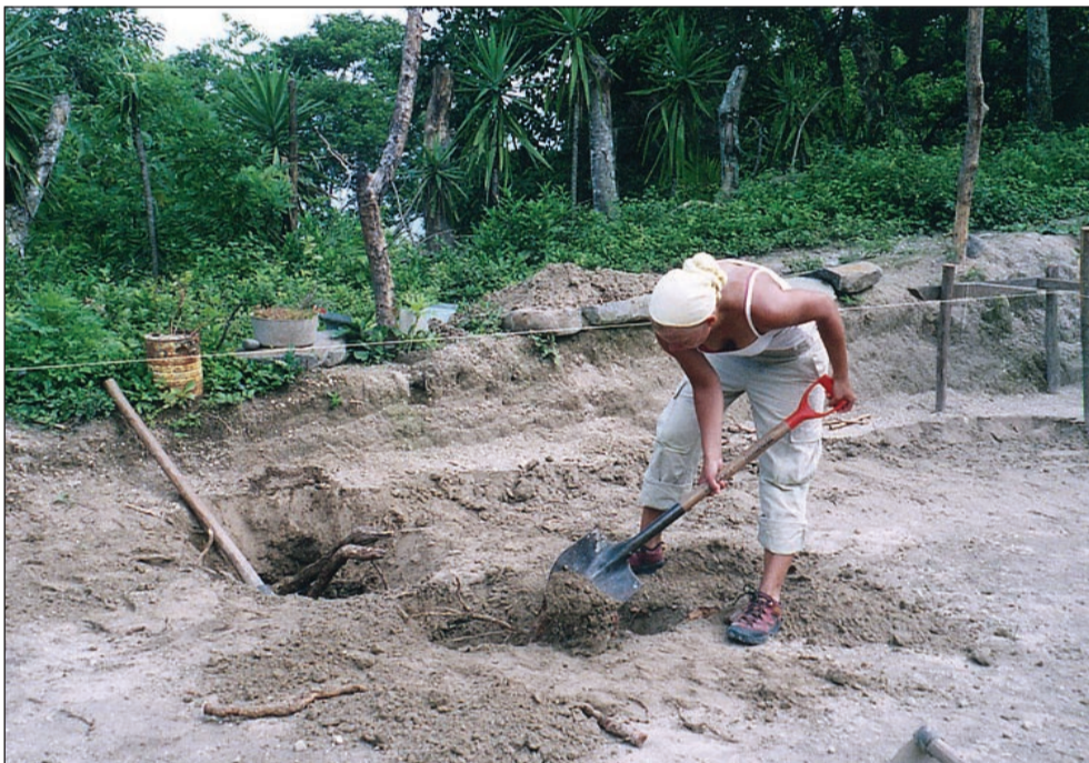
3. Prepare the ground: dispose of any tree roots, bones, remnants of abandoned latrines etc discovered. Excavate the area to be built on
