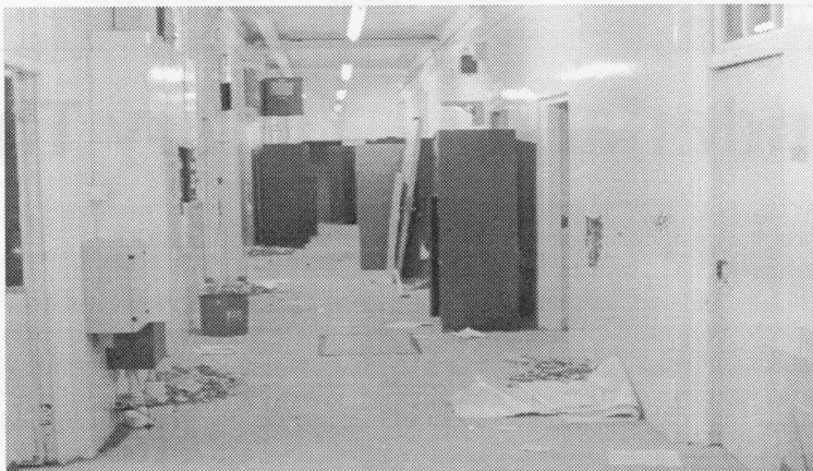
Photo: Jonas The East Wing basement as it presently stands - not a pretty site.
